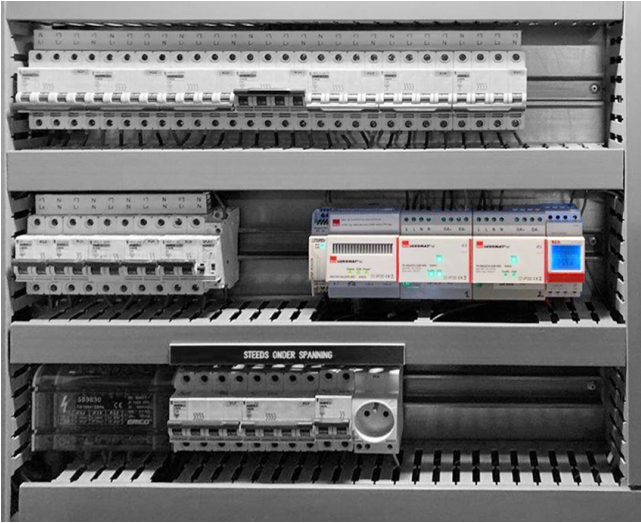
The system equipment, such as routers, power supplies, etc., has been reinstalled in the control cabinet.
