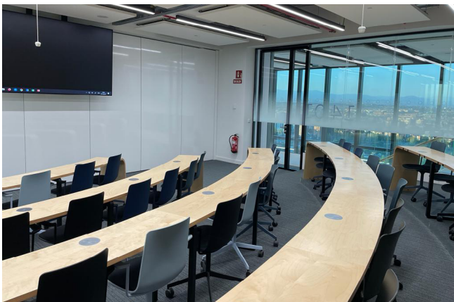
One of 64 multi-purpose classrooms fitted with B.E.G. KNX push-buttons (PB4-KNX-ST)
